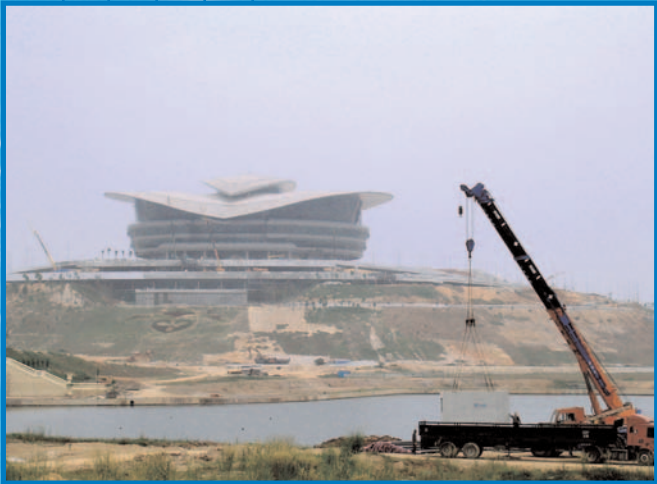
Putrajaya under construction with an Ecosol RSF 4600 unit in the foreground ready for installation.
