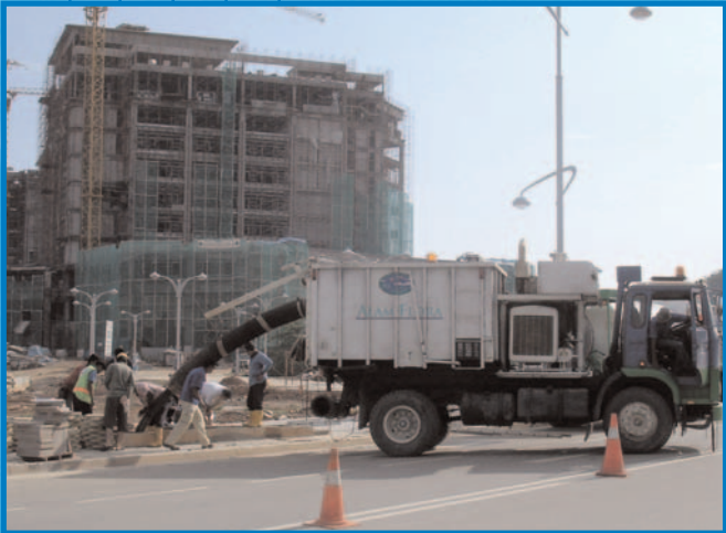
An Ecosol RSF 4600 unit being cleaned at Putrajaya. Over 2.5 tonnes of pollutants were removed.
